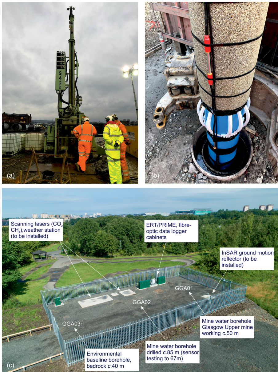
Fig. 5. Images of (a) drilling of the cored borehole GGC01 in 2018 and (b) installation of uPVC casing screen to mine water borehole with pre-glued gravel pack, electrical resistivity sensor cable (red sensors) and fibre optic cable. (a, b) BGS©UKRI 2020. (c) Research compound Site 1 at July 2020, background photograph courtesy BAM Nuttall.
