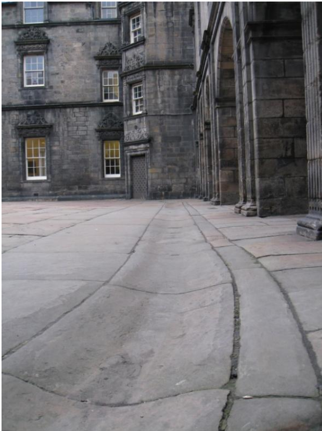
Fig. 26. Details at edge of central courtyard showing dished gutter with outer kerb, all made from Hailes-type sandstone. The kerb blocks are bedded on edge. George Heriot's School (1023)
