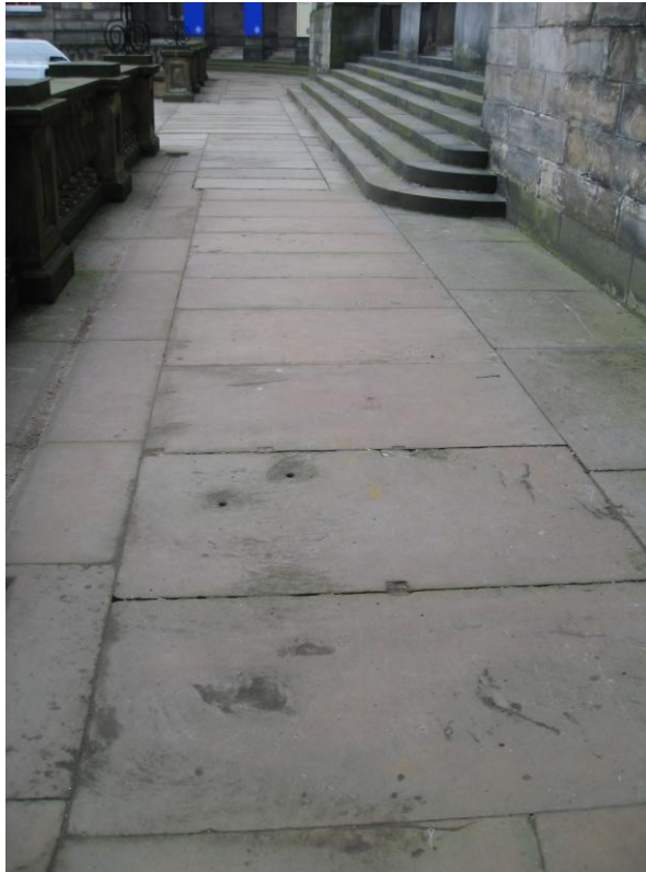
Fig. 1. Terrace pavement at west end of Old College, showing area of replacement paving with new slabs immediately adjacent to the steps. The terrace pavement and the steps below to the courtyard are replacement 'York-type' sandstone. Note the visual disruption to the original paving pattern where the new slabs have been inserted (3062).
