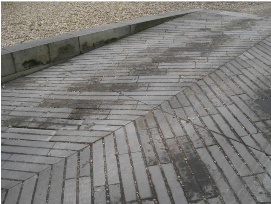
Fig. 45. Vehicle access area executed using elongate sandstone blocks, showing coarse tooling to mimic the historic sandstone setts at entranceways to historic Playfair paving schemes. National Galleries (3144)
