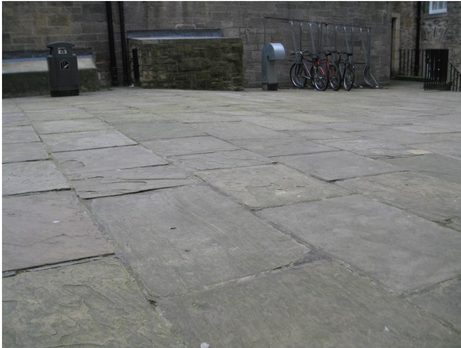
Fig. 38. Sandstone paving, probably re-laid in the 1960s, showing the typical variable appearance and natural 'contoured' surface texture typical of local sandstone such as Hailes. Milne's Close (909)
