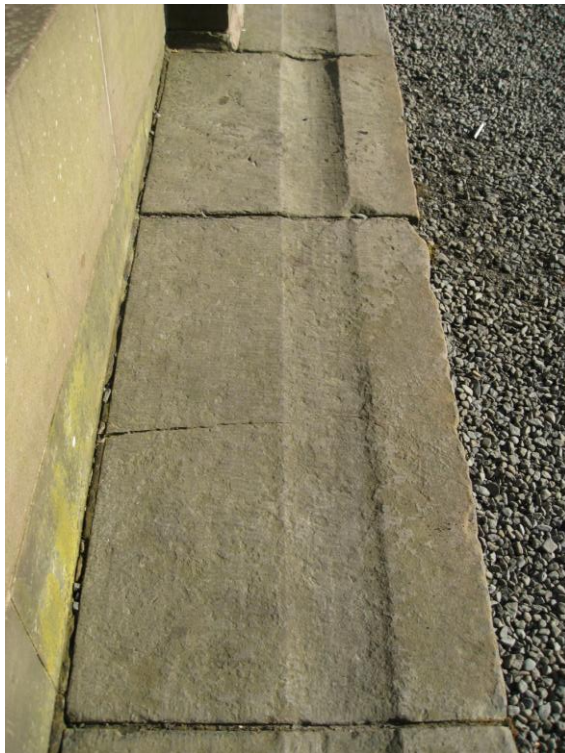
Fig. 9. Detail of 'original' dished sandstone gutters at base of terrace wall adjacent to gravel of central courtyard (east end), showing traces of the original broached tooling. (3472)
