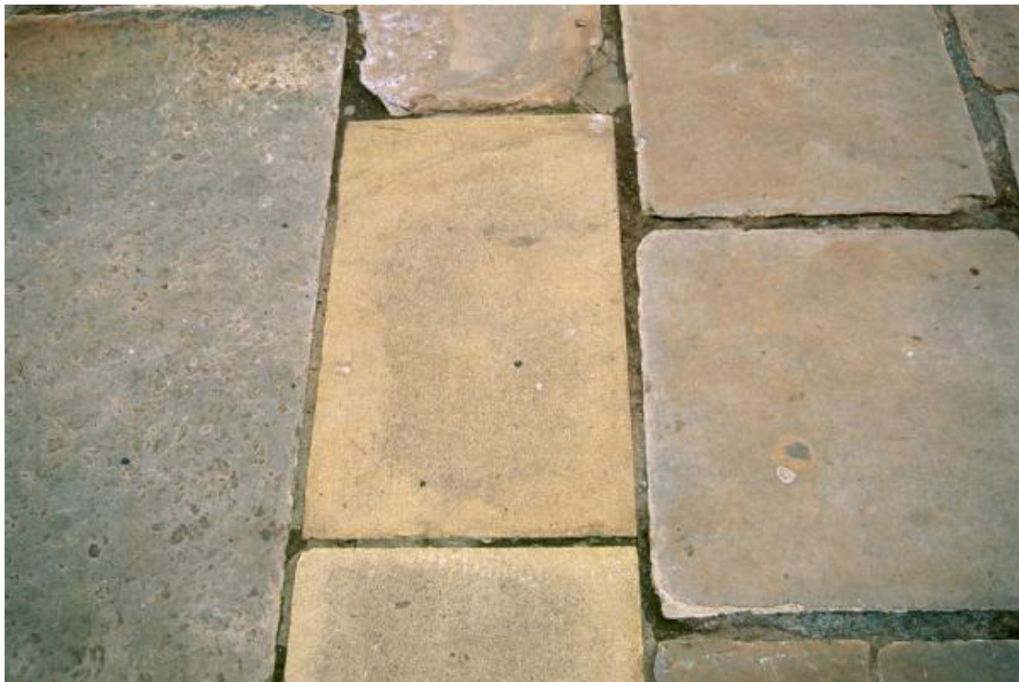
Fig. 49. Small area of modern replacement paving in Charlotte Square, with two slabs of York-type sandstone (centre of image) showing typical uniform, strong yellow-buff appearance, contrasting with the original 'Hailes type' sandstone (to either side) showing a more variable appearance ranging from grey to orange-brown colour.
