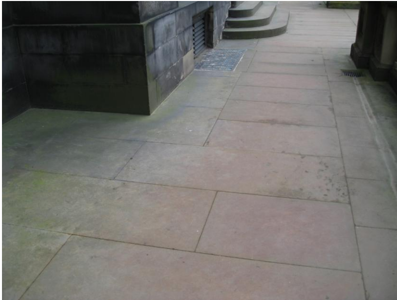
Fig. 7. Transition between wide pavement area and narrow area. Note continuation of the paving pattern with edge courses at each side (dished gutter to balustrade on right-hand side), and single central slab laid perpendicular to pavement direction. Note the regularity of slab sizes (3075).
