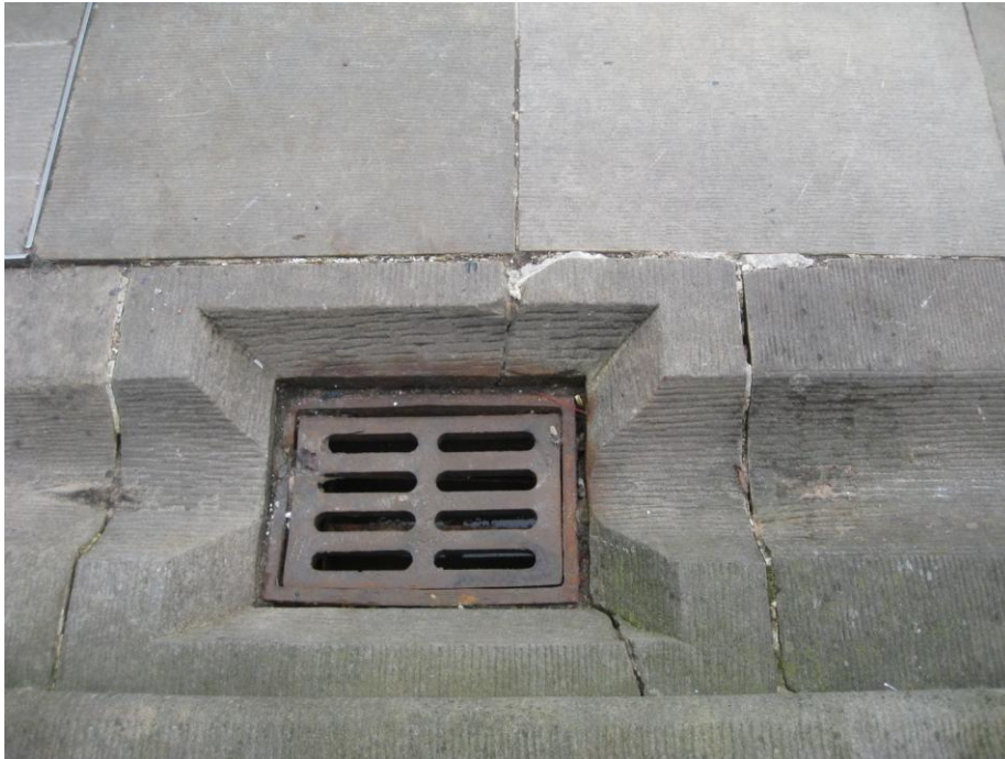
Fig. 44. Well executed masonry detailing around drain in dished gutter in recent paving using Clashach sandstone. Note traditional fine droved tooling finish, replicating that seen on original historic sandstone paving in Playfair schemes. National Galleries (3140)
