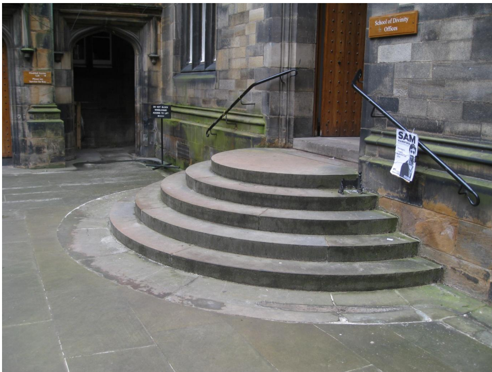
Fig. 32. Curved entrance steps of Hailes-type sandstone showing variable colours with orange-red patina, adjacent to replacement paving in courtyard which is a more uniform 'York-type' sandstone. New College (3102)
