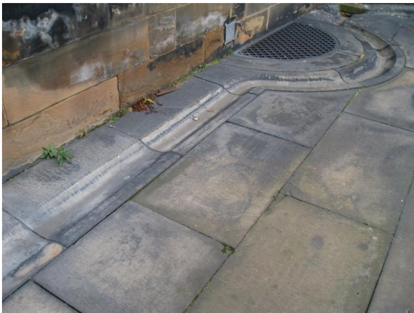
Fig. 18. Drainage channel at edge of main courtyard, showing dished gutters cut into single sandstone blocks. The depth of the cut channel varies along the length of the gutter to control water flow (here deepening from left to right). Note curved detail around ventilation grill. Donaldson's Hospital (3205).
