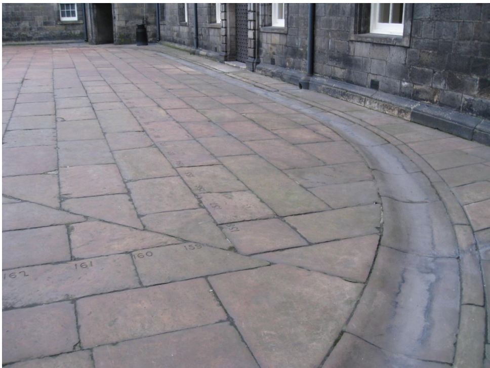
Fig. 22. Details of corner in central courtyard showing radial linear junction and curved dished gutter at corner. George Heriot's School (3251)
