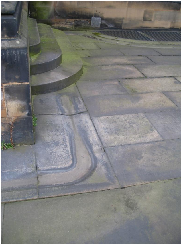
Fig. 17. Drainage channel and step edge detail at perimeter of main courtyard, showing dished gutters cut into single sandstone blocks. Donaldson's Hospital (3214).
