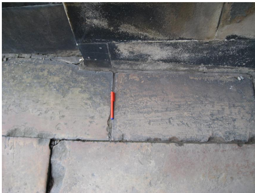
Fig. 10. Remnants of surface tooling on paving, generally preserved only in areas of low footfall or adjacent to buildings. The tooling consists of a series of narrow rows of fine droving running across the slab. In most places the tooling has worn away, although the grainsize of the sandstone gives the stone a natural slip resistance. (3051)
