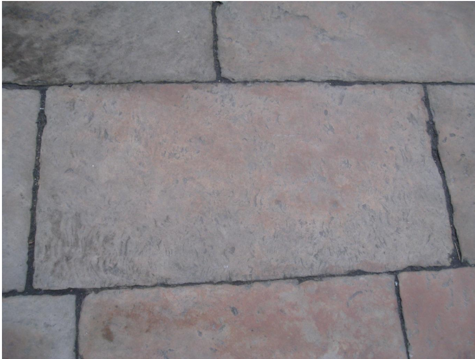
Fig. 21. Detail of paving slab showing orange-brown patina and 'contour-bedded' surface characteristic of Hailes type sandstone. George Heriot's School (3245)
