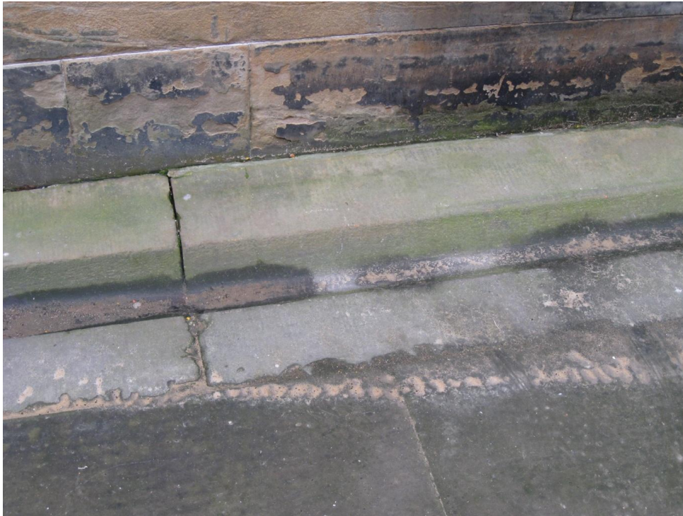
Fig. 31. Remaining section of original dished sandstone gutter at edge of replacement paving to courtyard. Note the finely tooled (droved) surface finish. New College (3099)
