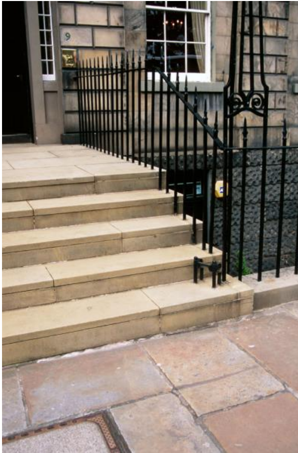
Fig. 50. Use of replacement Yorkshire sandstone as replacement steps adjacent to original 'Hailes type' sandstone paving (Charlotte Square). The typical uniform yellow-buff colour of the York stone contrasts with the more variable and stronger coloured original paving slabs. Note also the poor detailing of the replacement steps, particularly the use of a thin slab.
