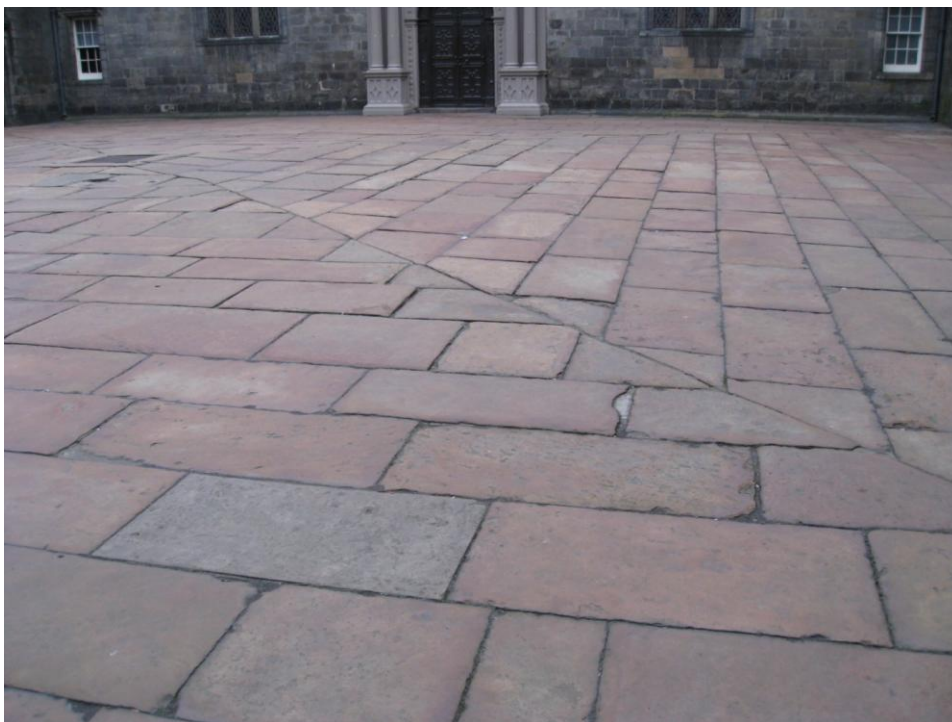
Fig. 20. General view of central courtyard showing rectangular centred paving pattern with diagonal linear joins at corners. The flagstone is Hailes-type sandstone showing a characteristic orange-brown patina with 'contour-bedded' surface. George Heriot's School (3247)
