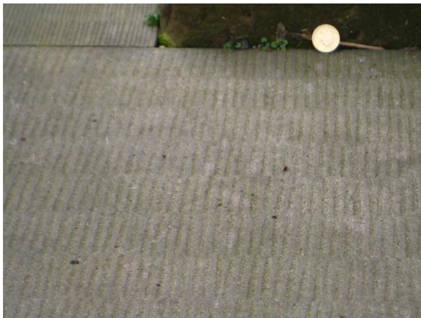
Fig. 41. Detail of surface of replacement Clashach sandstone paving slab, showing hand-tooled droved surface finish, similar to those observed on well preserved examples of original sandstone paving at other Playfair sites. National Galleries (949)
