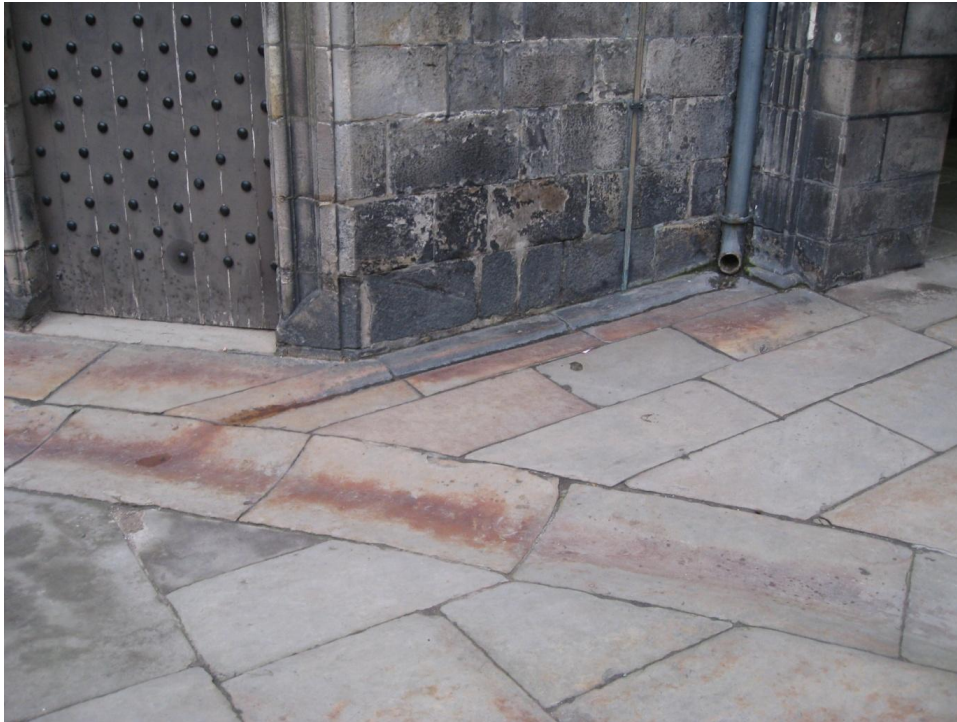
Fig. 25. Edge of central courtyard at north entrance showing main curved dished gutter with adjoining smaller gutter from downpipe outlet, made from Hailes-type sandstone. George Heriot's School (3242)
