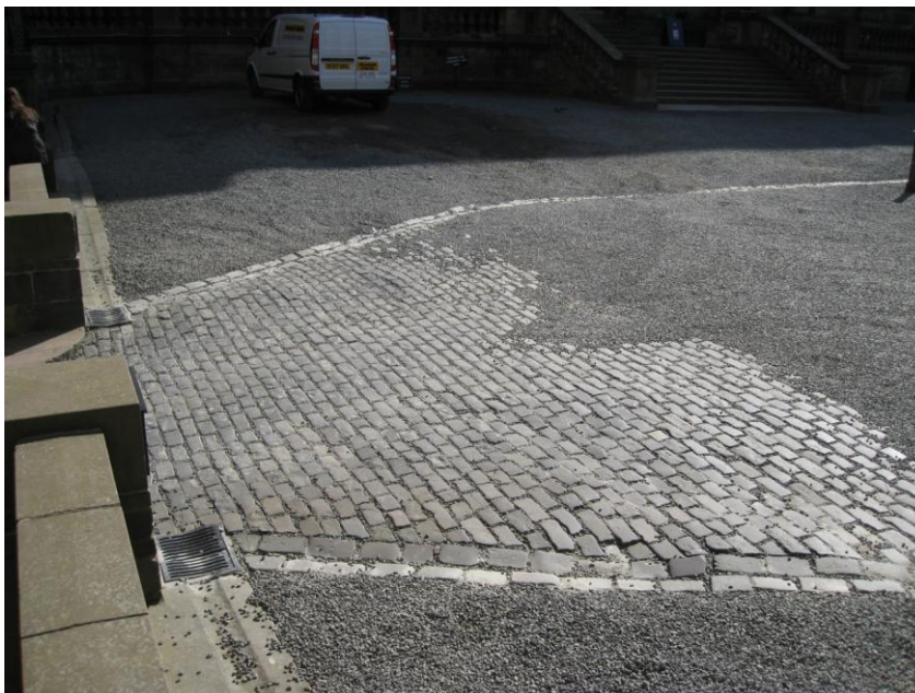
Fig. 12. Inner vehicle entrance to Old College, comprising dark whinstone setts leading to the gravel courtyard. (3430)
