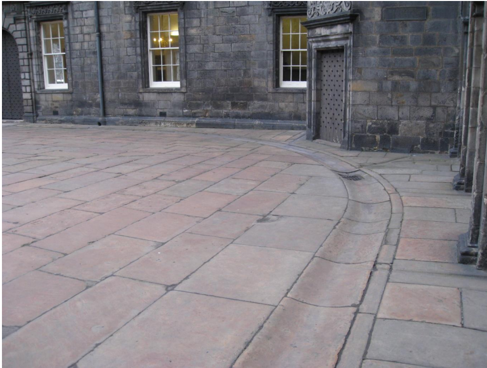
Fig. 23. Detail of corner in central courtyard showing curved dished gutter at corner. George Heriot's School (3235)
