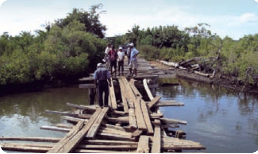
All in a day's work! Negotiating a river crossing damaged by floods in northern Madagascar.
