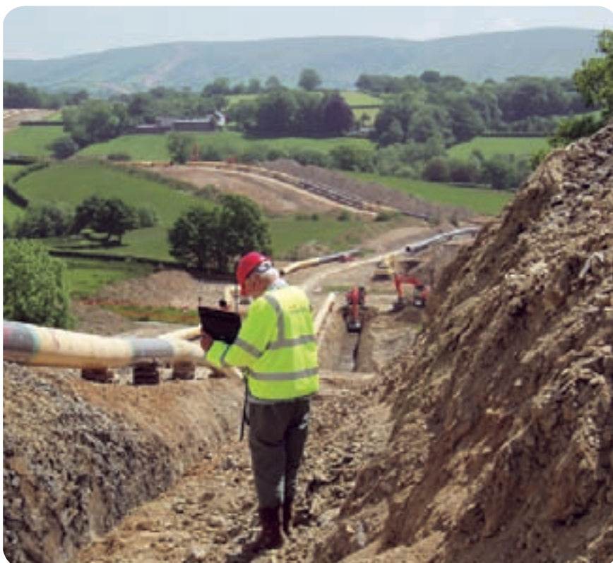
A BGS geologist observes rocks exposed in the gas pipeline trench excavated near Llandovery, mid Wales.
