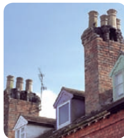
Chimney damage, Gainsborough, caused by the Market Rasen earthquake.
