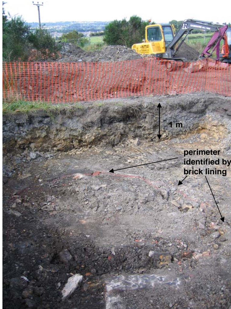
Plate 1 Backfilled mineshaft identified by brick lining approximately 3 m in diameter under approximately 1 m of spoil cover.
