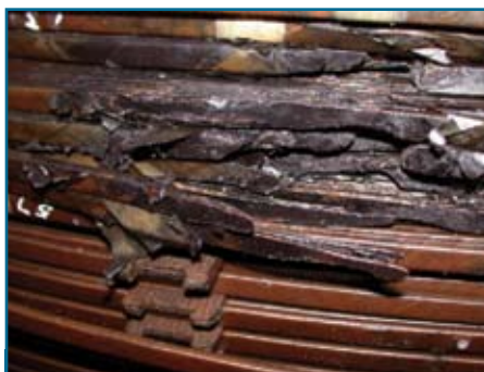
1: Failure in a large South African generator transformer, three weeks after the Halloween storm of 2003. The disruption of the winding and insulation by the arcing fault at the time of final failure is clear. The arcing fault also destroys evidence that might lead to a better understanding of the progression of damage after initiation by the geomagnetic current event. (From Thomson et al. 2010)
