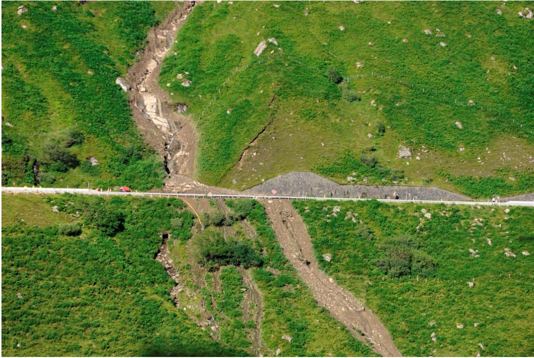
Figure 7 The debris flow path above and below the A83 Rest and Be Thankful pass in August 2012
