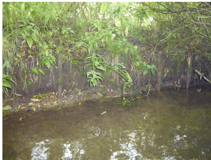
Figure 3.3.3 Remnants of wooden bank reinforcement
