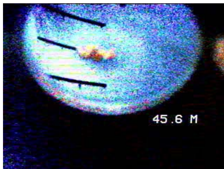
Figure 5. Screen slots and iron bacteria in the Gayo borehole
