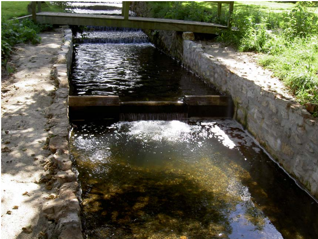
Figure 2 Photographs of partially completed fish pass and step structure at Tadnoll Mill
