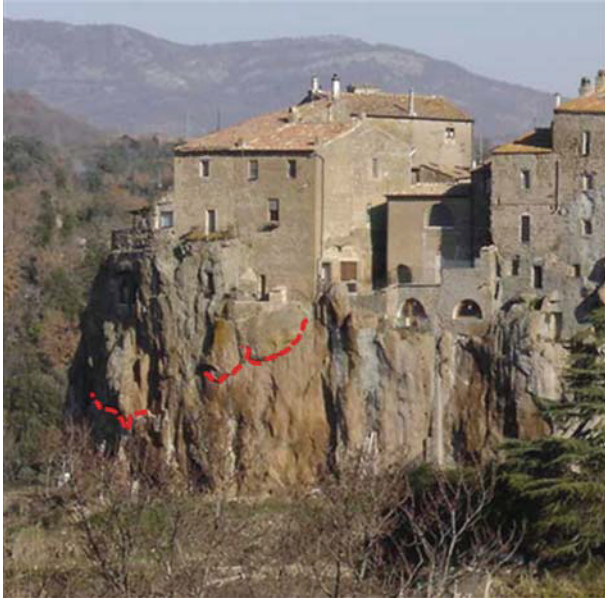
FIGURE 8: Detailed view of the south-western corner of the Pitigliano cliff. Close examination of the rock surfaces highlights the boundaries of rock wedges underneath the masonry walls.
