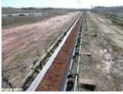
Photo 12. Sand and gravel conveyor
