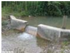
Photo 16. Clean water discharge
