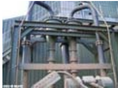
Photo 34. Washing plant cyclones
