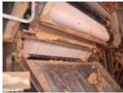
Photo 20. Belt filter press discharge
