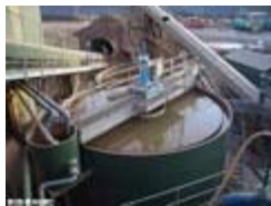
Photo 35. Washing plant thickeners
