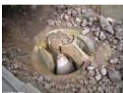
Photo 7. Primary Gyratory Crusher
