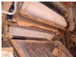
Photo 47. Belt filter press discharge
