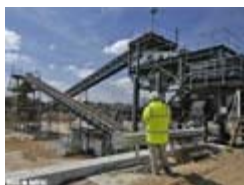
Photo 2. Sand and gravel washing plant
