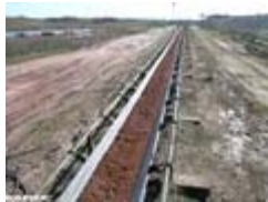
Photo 36. Sand and gravel conveyor
