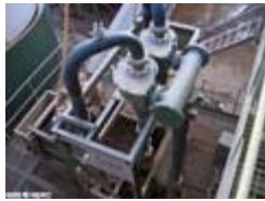
Photo 23. Washing plant cyclone
