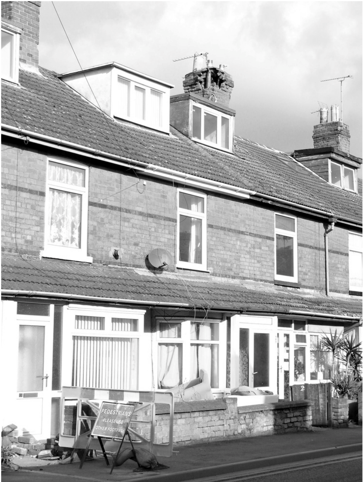
Figure 3 - Street scene in Gainsborough on the day of the earthquake, showing an instance of chimney damage (BGS photo by SL Sargeant; see also cover picture).
