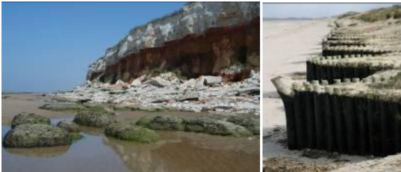
Erosion at Hunstanton Cliffs (left) and erosion defences at Brancaster (right). Both photos supplied by Environment Agency
