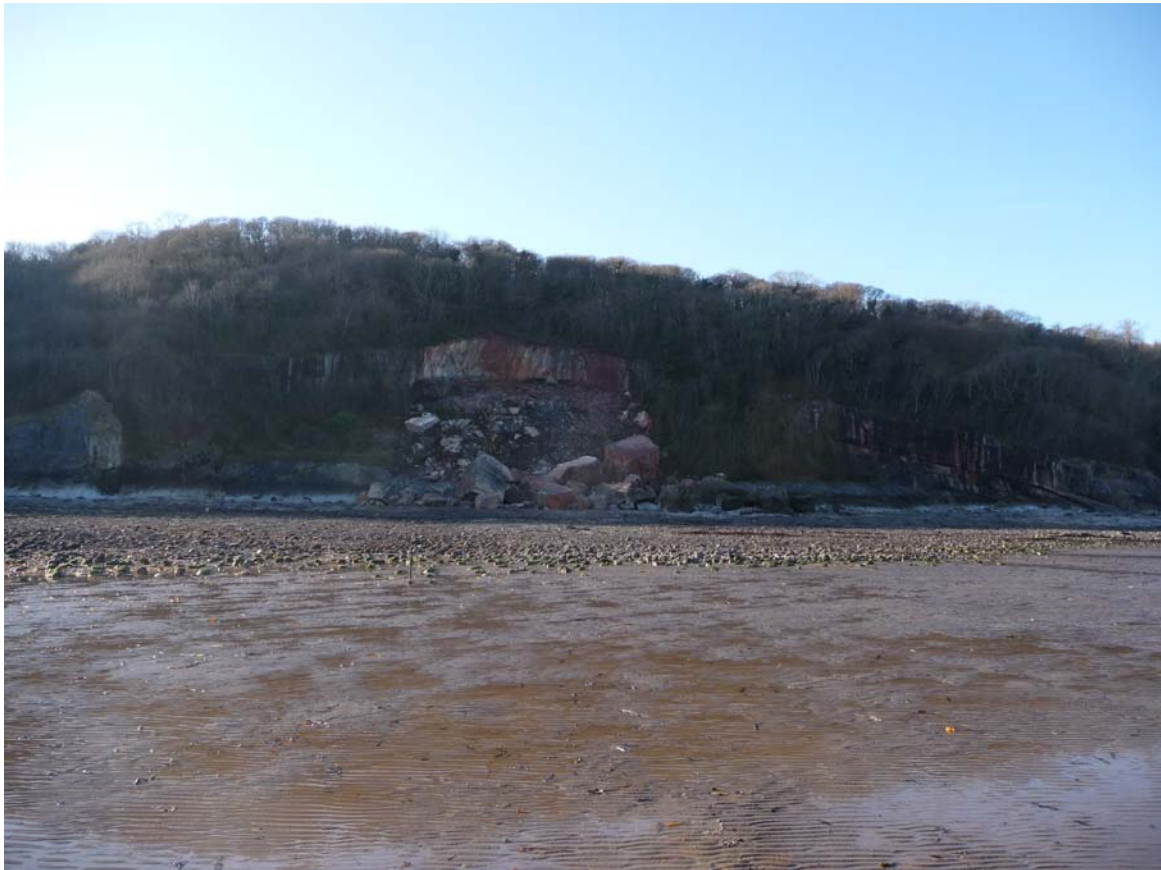
Figure 8. Wide angle view of the Oxwich Bay landslide showing its position within a disused limestone quarry. Photograph taken from NGR 250782 185968 looking west.
