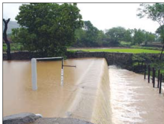
Photo A5.3 Water level monitoring equipment in CD3, flowing at full capacity.
