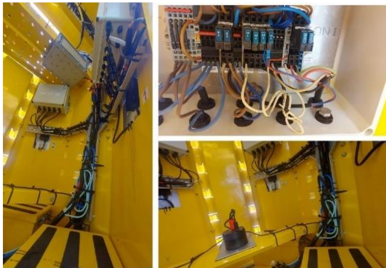
Cables inside the tower JC247 deployment
