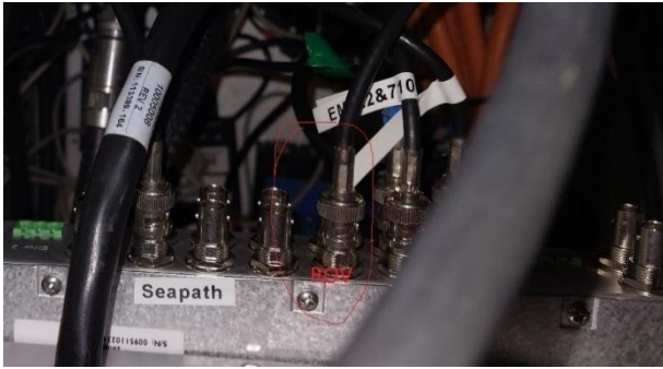
Fig. 7.109 Photo of BNC Coax in the Gyro Room, on the Seapath PPS distributor unit
