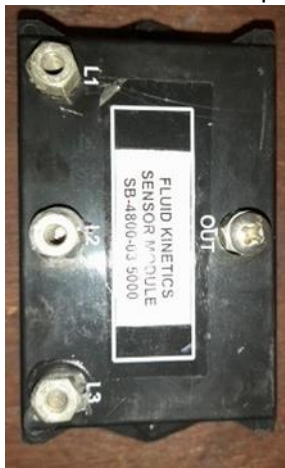
Fig. 7.113 Picture of the high voltage monitoring module
