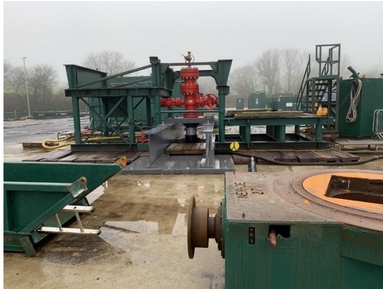
Figure 3: Geothermal drill site at the Eden Project, Cornwall, visited during the field campaign. The site was being prepared for pump tests with a new heat exchanger at the time of the visit. BGS © UKRI. All Rights Reserved.
