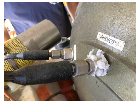
(c) Corrosion of aluminium connector adaptor between D.G. O'Brien Coax connector for Iridium/GPS antenna and anodised aluminium pressure vessel.
