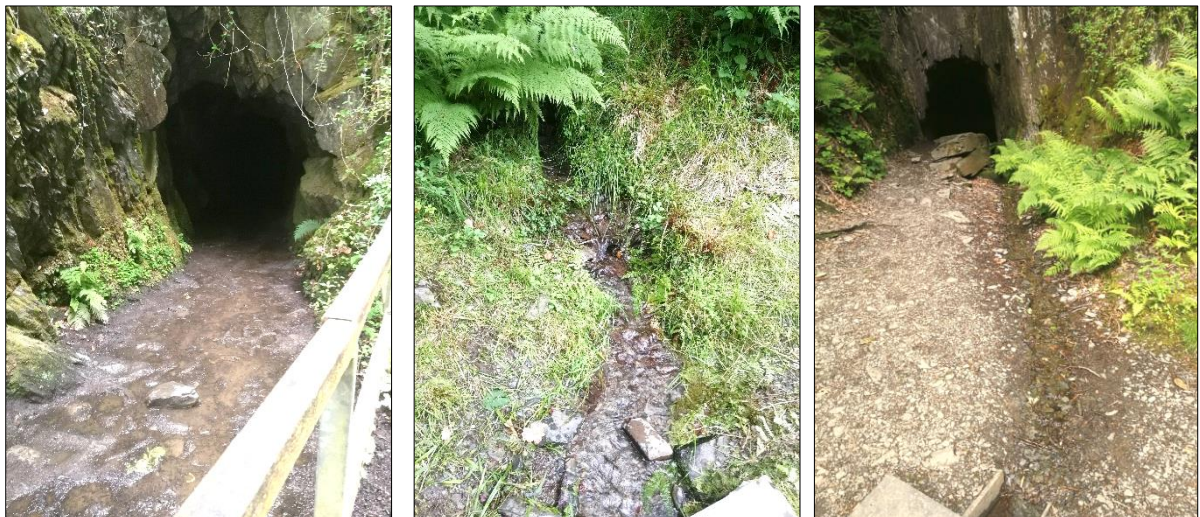
Figure 15: Entrance to adit 3 (left), drainage from hillside between adit 2 and 3 (centre) and entrance to adit 4 (right).
