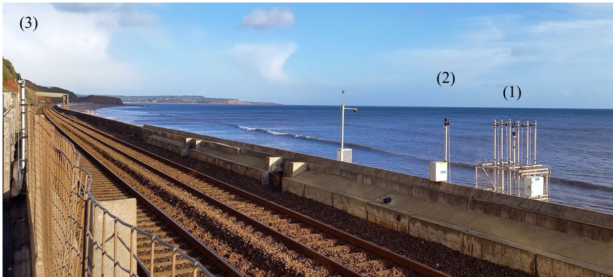
Figure 11. WireWall deployment at Dalwish (Devon, UK). A full WireWall (1) system is located at the crest of the sea wall, with two smaller WireWall systems located further inland on the seawards (2) and landwards (3) side of the railway tracks. Also visible is a B-SCAN system installed by the University of Plymouth to measure daily beach levels fronting the sea wall.
