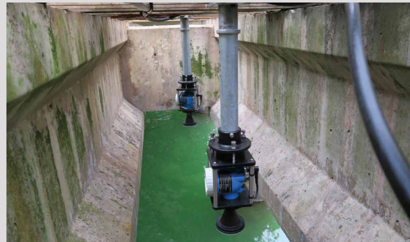
▲ Dual radar sensors installed by the NOC at Belize City beneath a jetty walkway, where they are safe from damage by shipping. (© Jeff Pugh, NOC)
