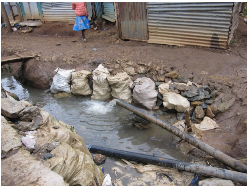
Figure 20 Mine water pumped directly into mining village culvert
