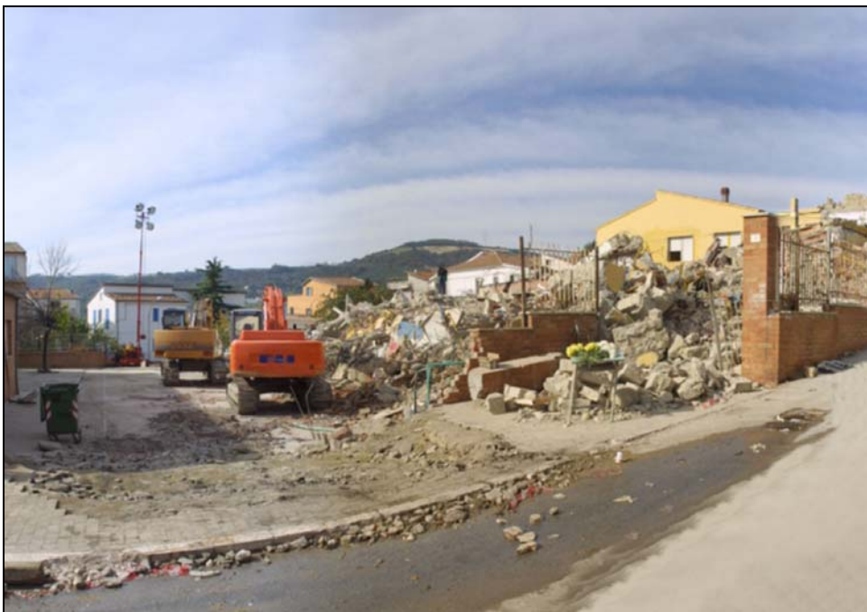
Figure 10. Aftermath of the magnitude 5.9 earthquake, Southern Italy on 31 October 2002. Photograph supplied courtesy of Dr. Romano Camassi, INGV.
