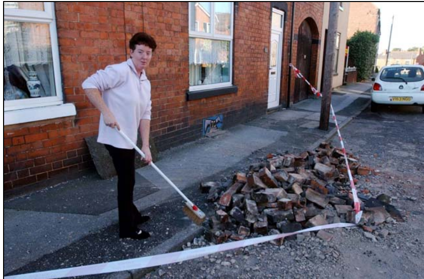
Figure 5. Damage to chimney observed after the Dudley earthquake. Photograph courtesy of PA Photos, London.
