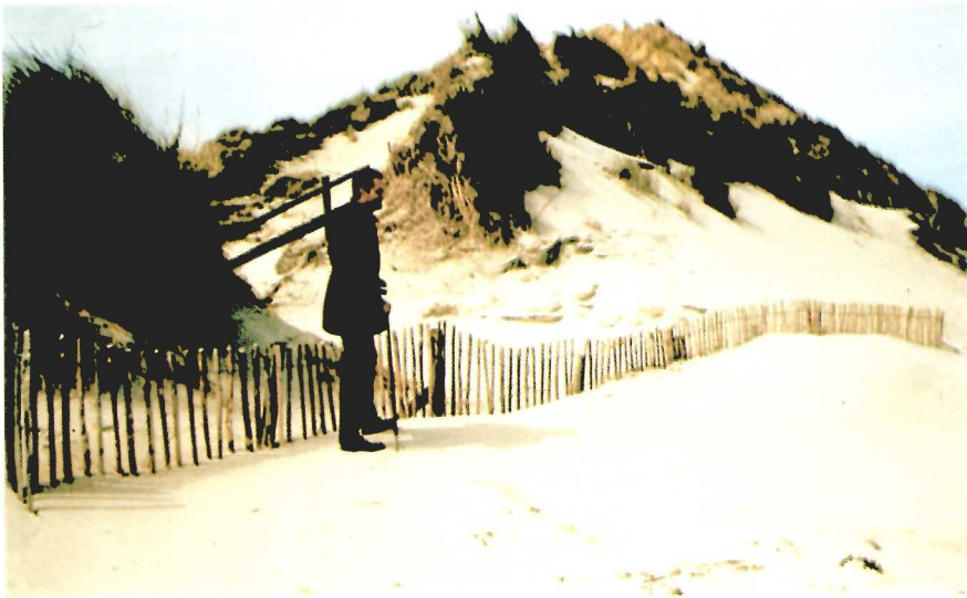
Plate 13. Wooden paling fences of 50% porosity are effective in trapping wind-blown sand. Gaps in the coast dune resulting from trampling can be quickly heeled with sand fences followed up by planting. Note parts of 1 m high fence almost buried only 2 months after fence erected. (Photograph M J Hudson, Nature Conservancy Council copyright)
