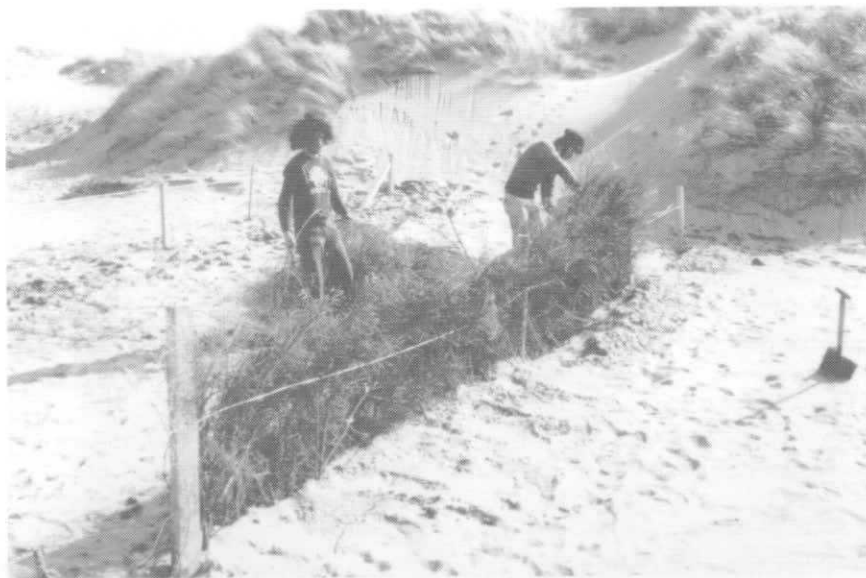
Plate 12. Physical aids are often needed to check erosion and accumulate sand in gaps in coastal dunes. Brushwood is a cheap material, ideal for building porous fences that are effective in trapping wind-blown sand. Natural materials of this kind also add valuable organic matter to the sand. (Photograph W T Band, Countryside Commission for Scotland copyright)
