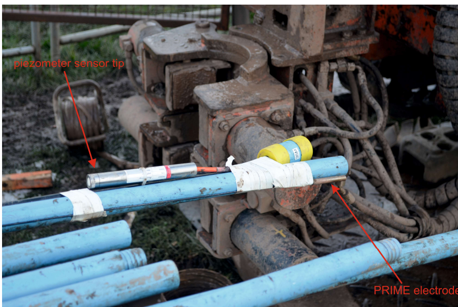
Figure 35 Lowermost PRIME resistivity array electrode taped to bottom section of sacrificial tremie pipe (blue) prior to installation in Borehole 3a
