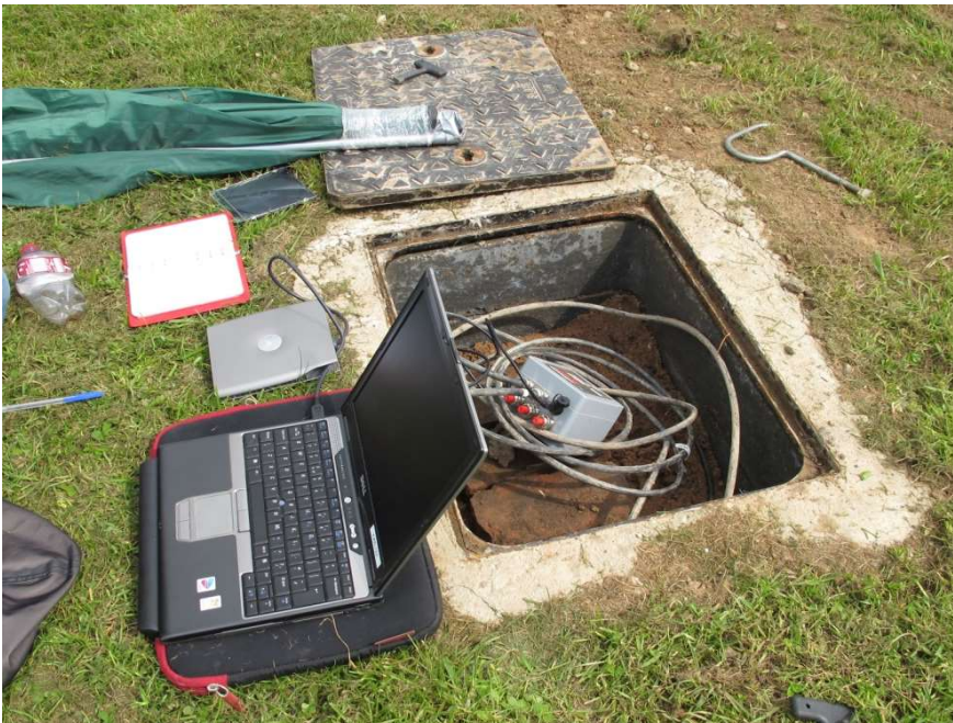
Figure 10 BGS monitoring piezometer arrays - Surface installation for piezometer arrays datalogger for boreholes 1a and 2a.
