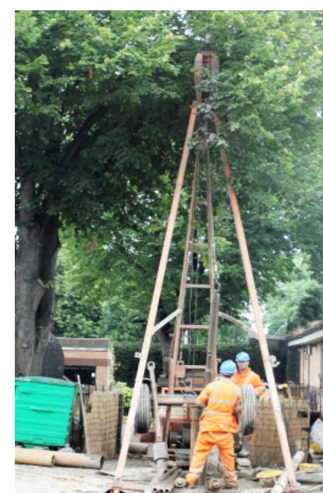
Fig. 4. Drilling the 18m deep abstraction borehole at the GSHP test site in Cardiff. The water table is 4m below surface.
