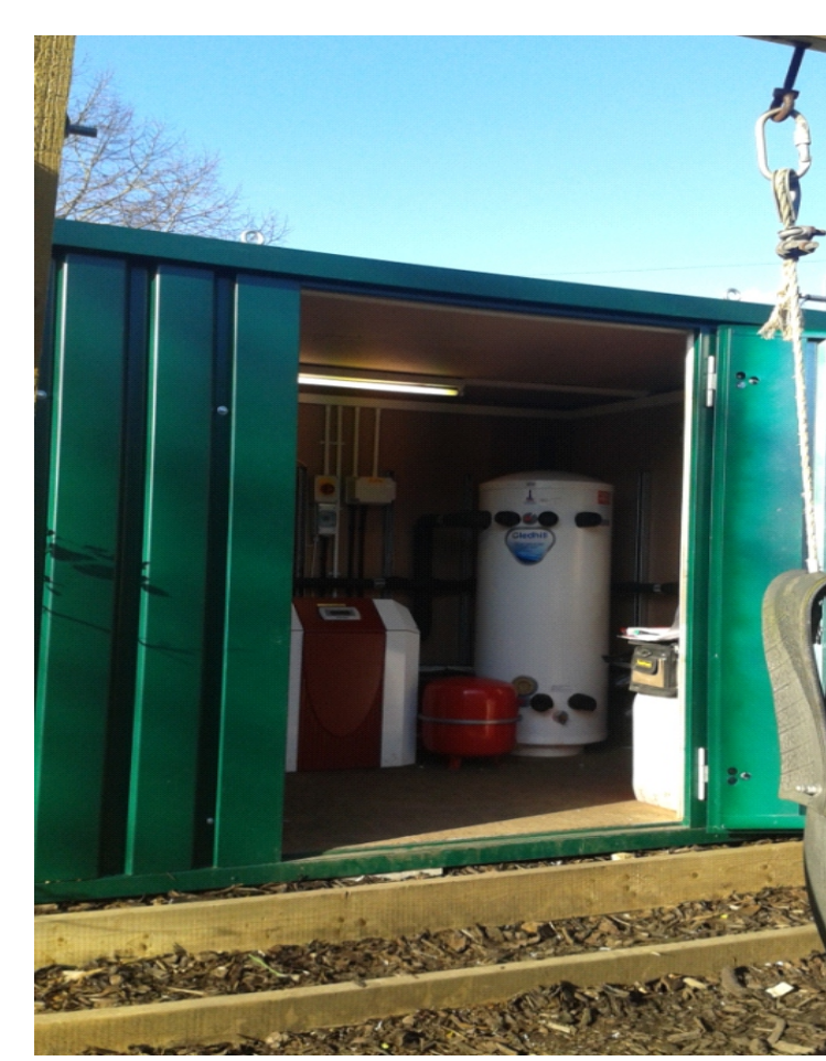
Fig. 6. Water-to-water heat pump test rig (2x 11KW units) housed in portable container, located in the school garden.
