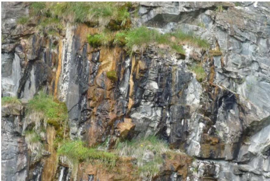
Figure 9 Groundwater seepage from discrete fracture in quarry face
