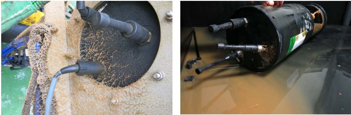
Figure 23 - Broken connector of the CO2 sensor at the frame
