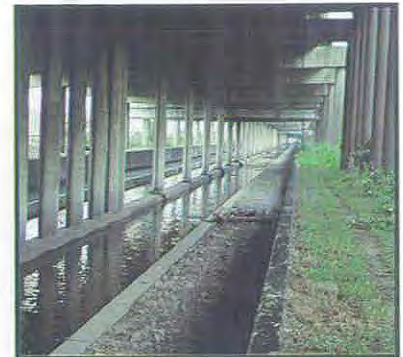
Heavily channelised section of the River Tame, West Midlands, running below the M6.
