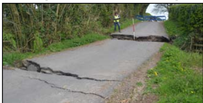
Figure 6. Reactivated landslide in Herefordshire (photo: BGS).
