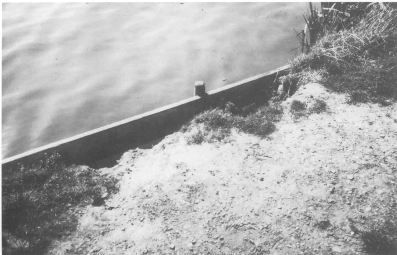
Plate 7. Erosion effects on bankside habitat, before and after reinstatement: i. eroded river bank used by coarse anglers
