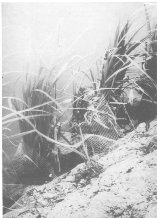
Plate 8. Plantings of greater pond-sedge ( Carex riparia ) into woven geotextile 'pocket' fabric for canal bank protection and habitat improvement purposes (Photograph British Waterways Board)
