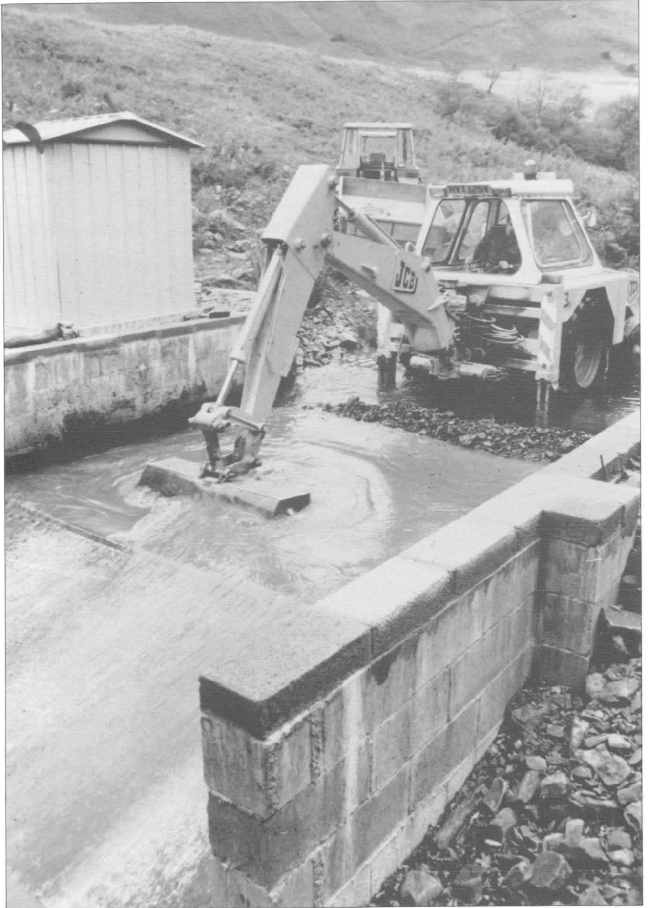
Plate 5. Flood events can result in considerable transport of bed-load sediments. Emptying trapped bed-load sediment from the Crump weir at the lower end of the Afon Cwm, Llanbrynmair (Photograph G J L Leeks)
