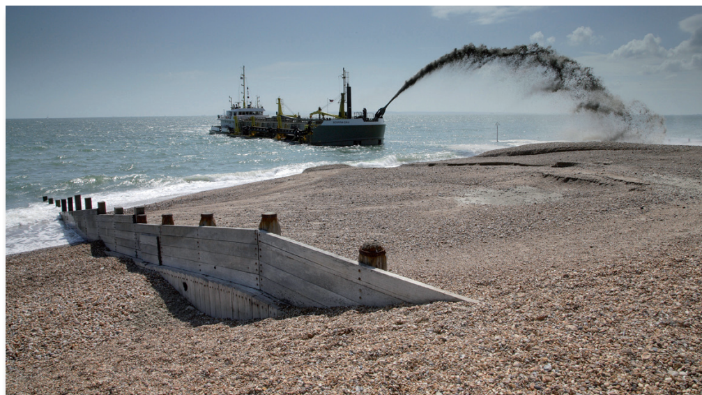
Figure 10 Beach nourishment with marine dredged sand and gravel — Hayling Island © Westminster Dredging.
