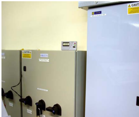
Plate 4: SNS Server Room (Near Door)
